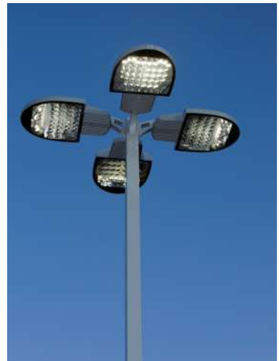
Outdoor LED Lighting Array
